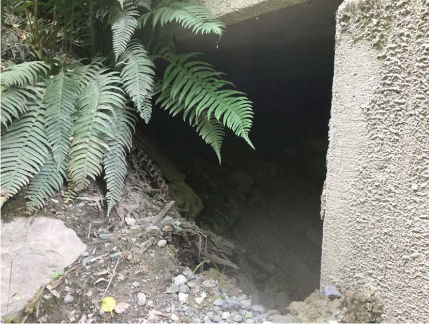
Loosing fill behind RB cap
